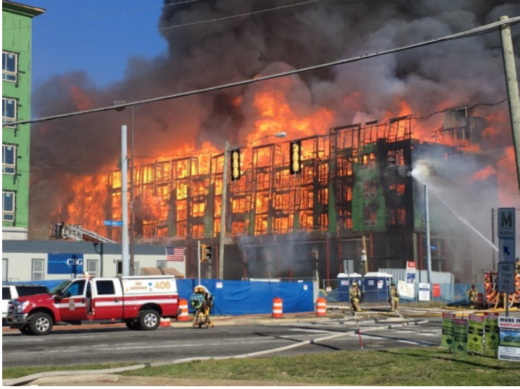
Virginia firefighters battled a large fire at a multistory construction site in Fairfax County, Virginia. (Courtesy Anthony Kelleher)
